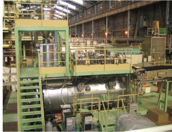
1200 kW EB melting furnace (example)
